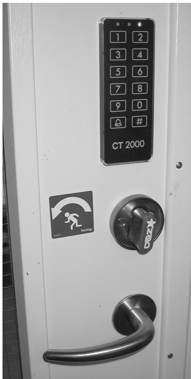
Figure 1. Biosecurity and safety measures collide at BSL-3 laboratory entrance. Safeguarding against access from intruders is ensured by the use of codes. The knob overrides the keypad, aiding access of rescue personnel in case of an emergency situation. The knob override is required to comply with safety regulations from Danish authorities.
